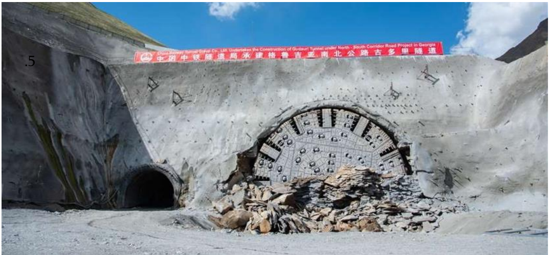
* The 9-kilometer Kvesheti-Kobi tunnel, the construction of which was completed on April 29, 2024.
